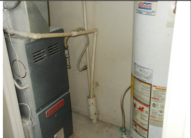
UNIT UTILITY ROOM
