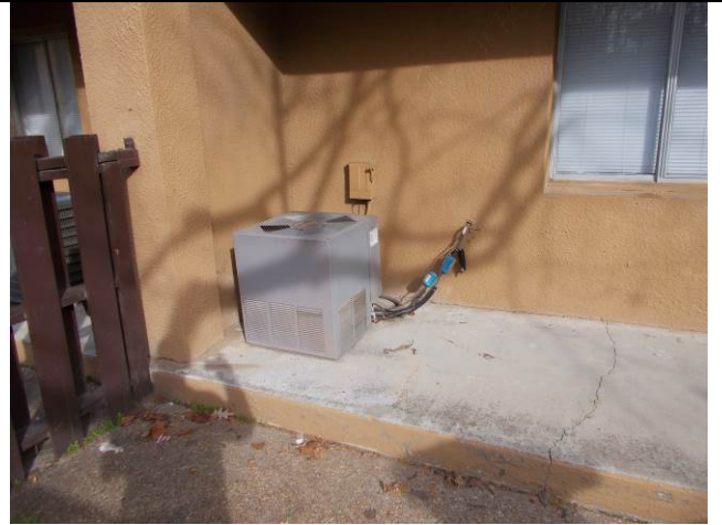
UNIT PATIO AND AIR CONDITIONING UNIT
