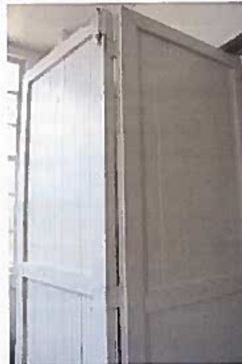
The Barney School's original wood partitions separate the two classrooms, providing more space for community use. Photo by Jeanne Cyriaque
