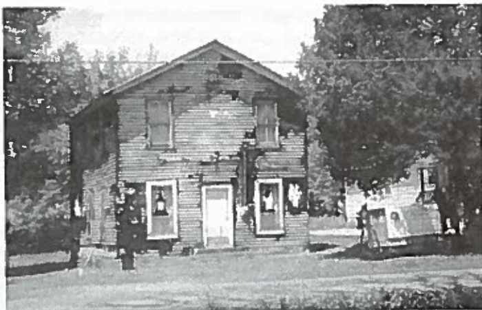
The preservation plan revealed several structural deficiencies and safety issues. The red asphalt siding was removed and revealed the original wood siding.
