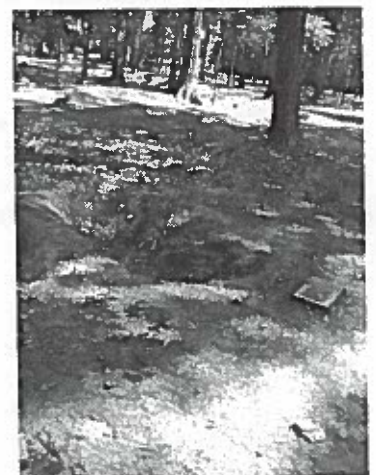
Sections of the School Street Cemetery contain deep depressions.
